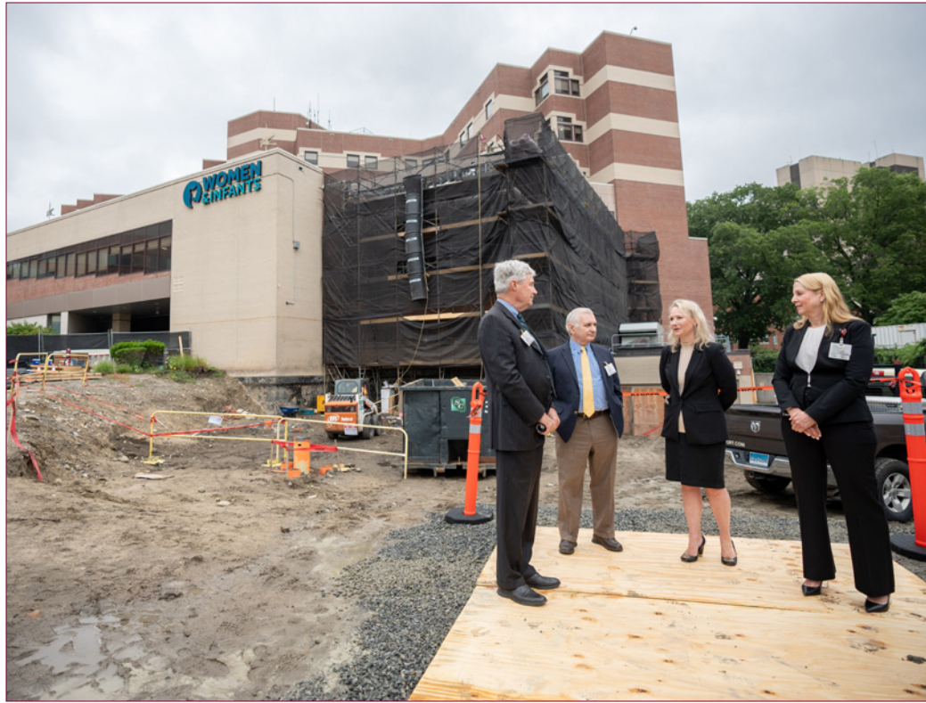
Shannon Sullivan , president and COO, of Women & Infants Hospital, toured the construction site of the new facility with Rhode Island Senators Reed and Whitehouse. [CARE NEW ENGLAND]
